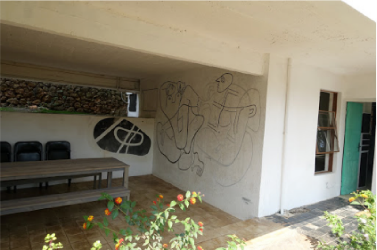
A bas relief mural by Le Corbusier has been carefully restored in the outdoor dining room.
